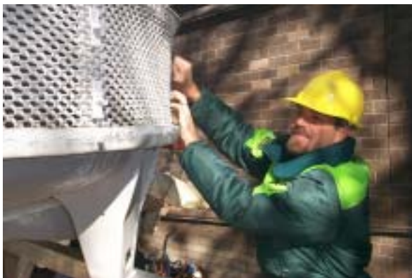
Left: Trade assistant Nathan helping to fit the air-conditioning cooling tower onto its support frame photo by Chris McCowage
